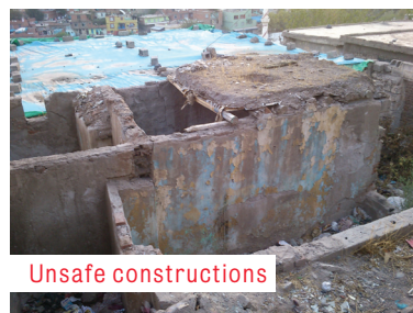
Poor sanitary conditions
