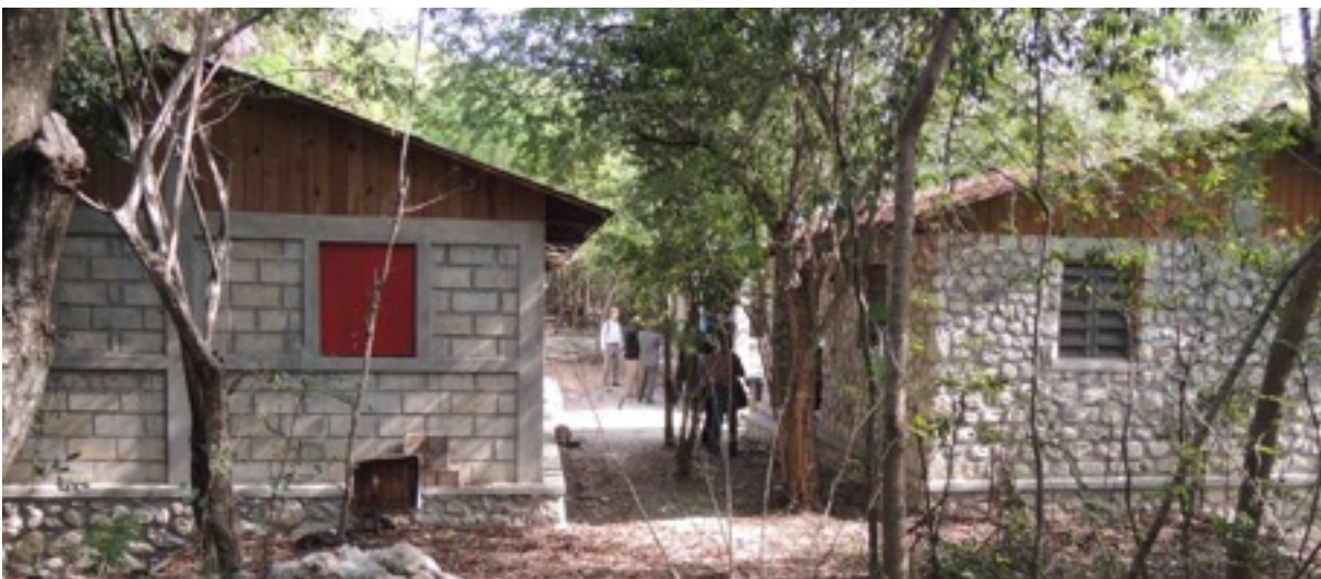
Reconstruction of homes post-earthquake, constructed under the guidance of ITECA (Institut de Technologie et d'Animation which has been active in Léogâne for over 30 years)
