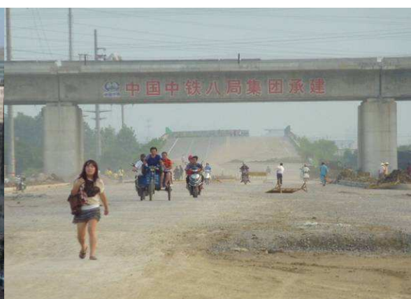
An expressway under construction below the new elevated Beijing-Shanghai high-speed railway line
