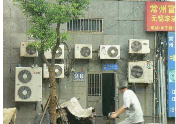
The energy efficiency issue
