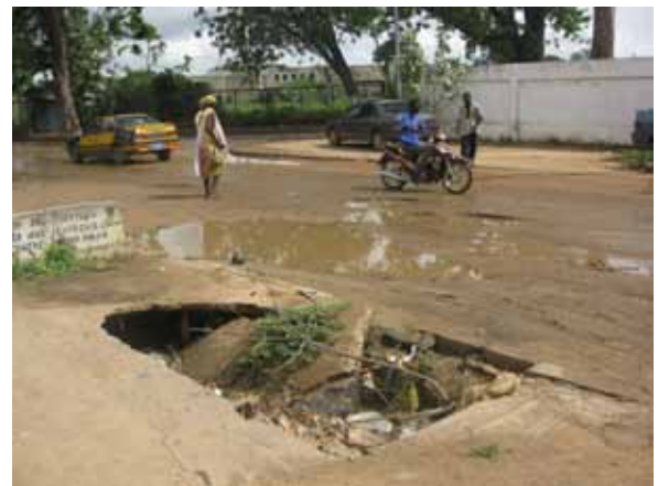
Pipes broken and filled with filth
