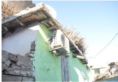
Airconditions in some houses
