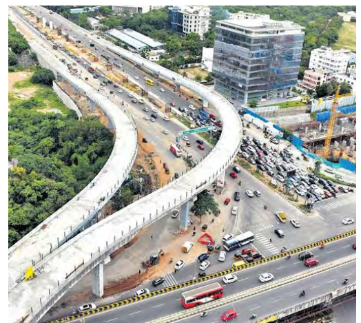
Construction of flyovers to keep pace with the increasing vehicle rush (source: Telangana Today)
