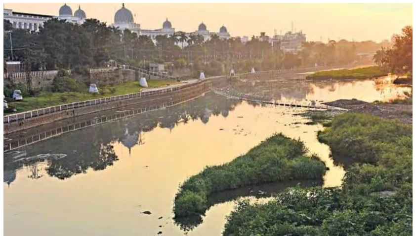
Ongoing Musi Riverfront Development along 55km of the Musi River in central Hyderabad (source: Telangana Today )
