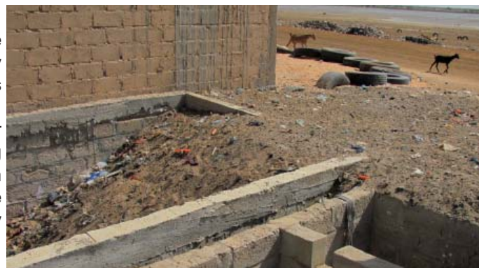
Foundation backfilled with waste - Pikine.
